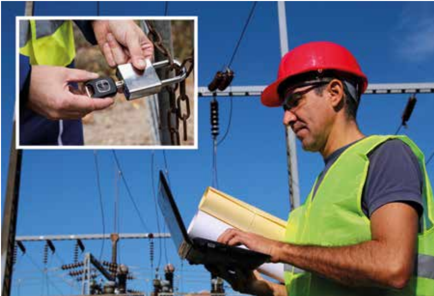
The Locken company provides first line access control for the electricity supply facilities and infrastructure of UK Power Networks (UKPN).
