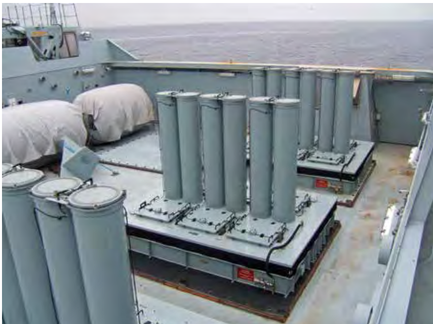
An example of a Standard Flex module: A Mk 56 vertical launcher module pictured here installed amidships on the Royal Danish Navy's ABSALON.
