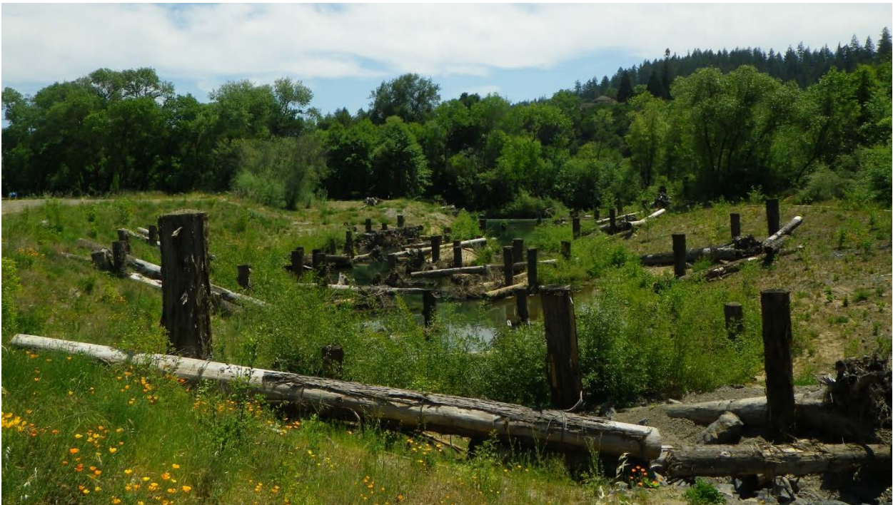
Figure 3.1.6. View of completed backwater pond habitat feature approximately 18 months after construction. Dry Creek Habitat Enhancement Demonstration Project, May 1, 2015.
