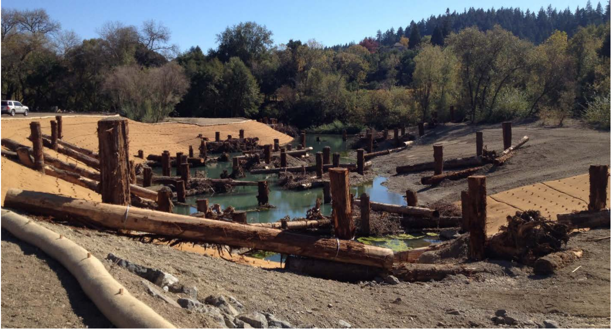
Figure 3.1.5. View of completed backwater pond habitat feature immediately after construction. Dry Creek Habitat Enhancement Demonstration Project, October 17, 2013.
