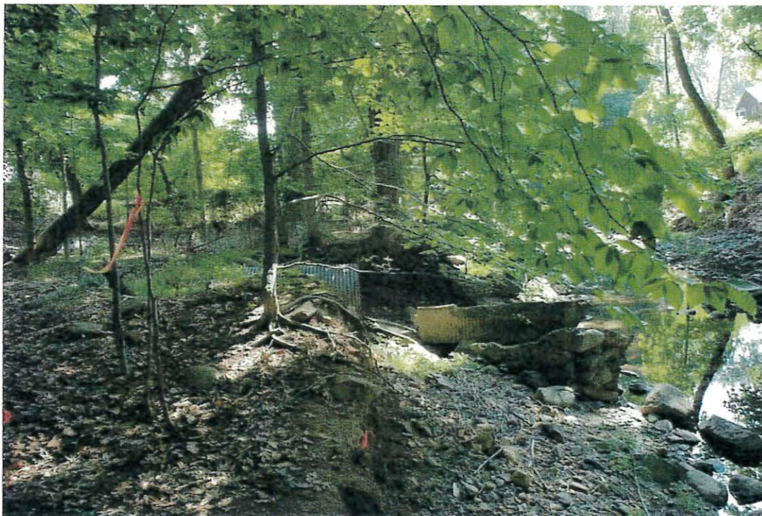
PHOTO #4 – View looking Southwest at the deteriorated storm sewer outfall structure nearest to plot/point OW-3. Photo Date: 07/12/2017.
