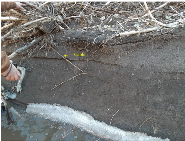
FIGURE 9 Loose cable allowed the revetment to float up during high discharges. Plumb Creek, KS [Color figure can be viewed at wileyonlinelibrary.com ]
