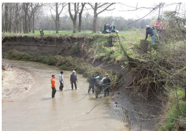
FIGURE 4 Construction of the cedar tree revetment on Wolfley Creek April 2017 (Nassar, 2019) [Color figure can be viewed at wileyonlinelibrary.com ]
