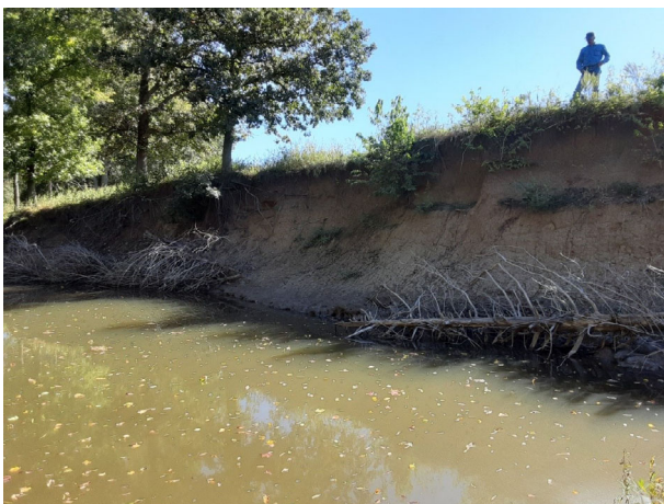
FIGURE 11 Cedar tree revetments have not captured sediment. One revetment is missing. Homer Creek, KS [Color figure can be viewed at wileyonlinelibrary.com ]
