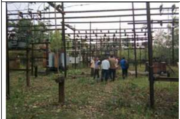
Photo 5: Existing Umrangso Substation
