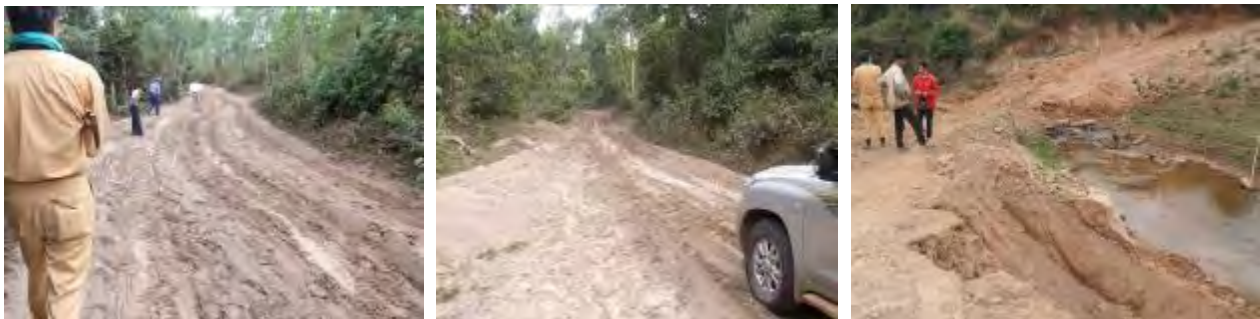
Figure-3 Road conditions in dry season before the Works
