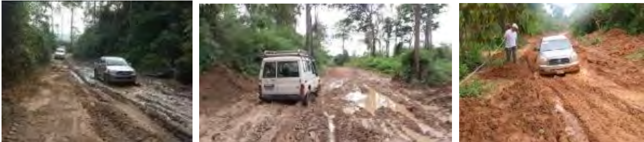
Figure-2 Road conditions in rainy season before the Works
