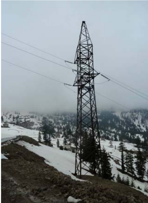
Figure 2.12: Existing 110 kV transmission line
