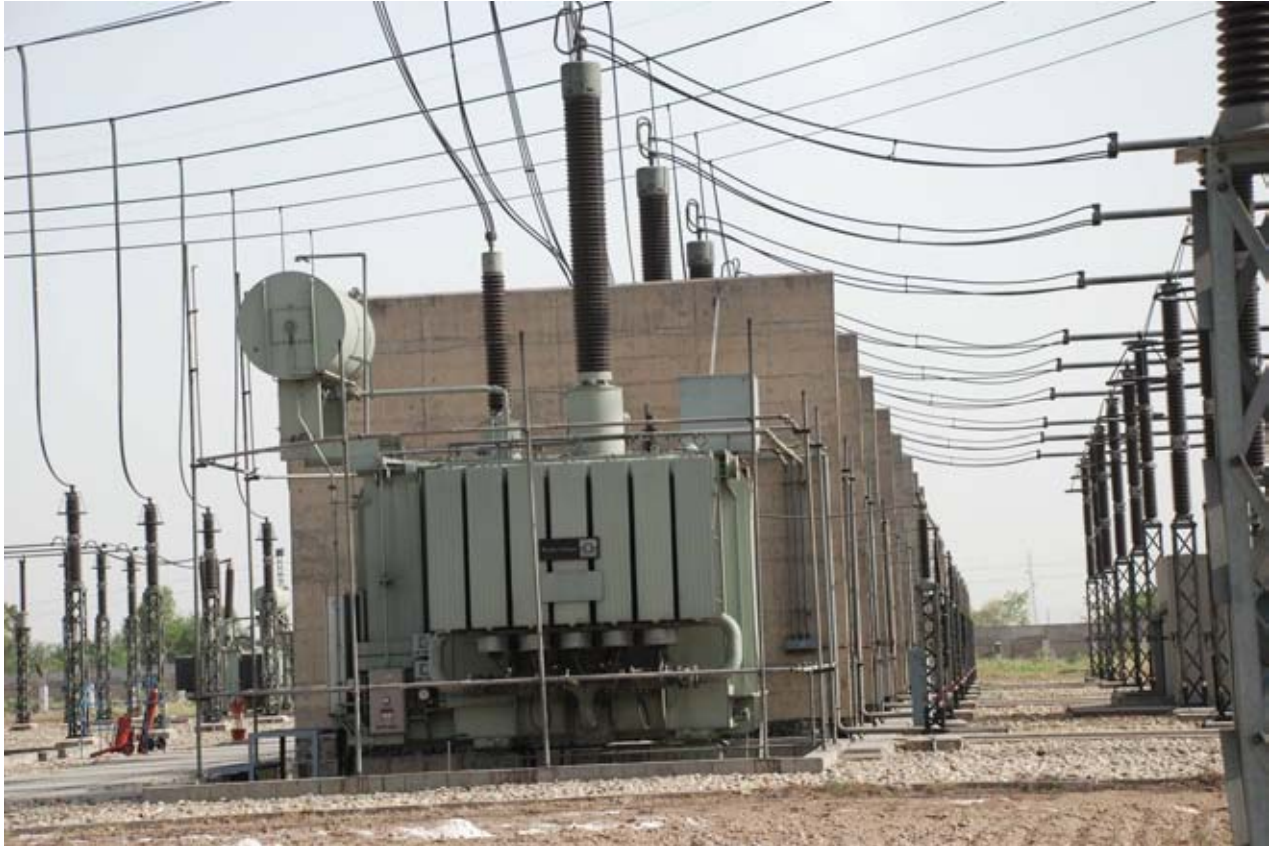
Figure 2.11: Example of Transformer and Switchyard location
