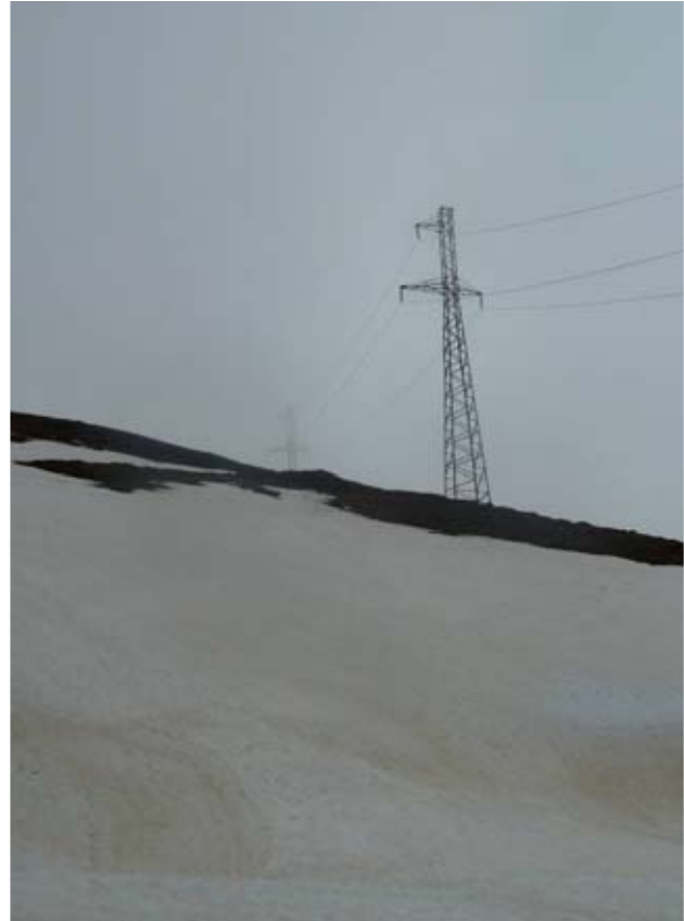
Figure 2.13: Existing 110 kV transmission line
