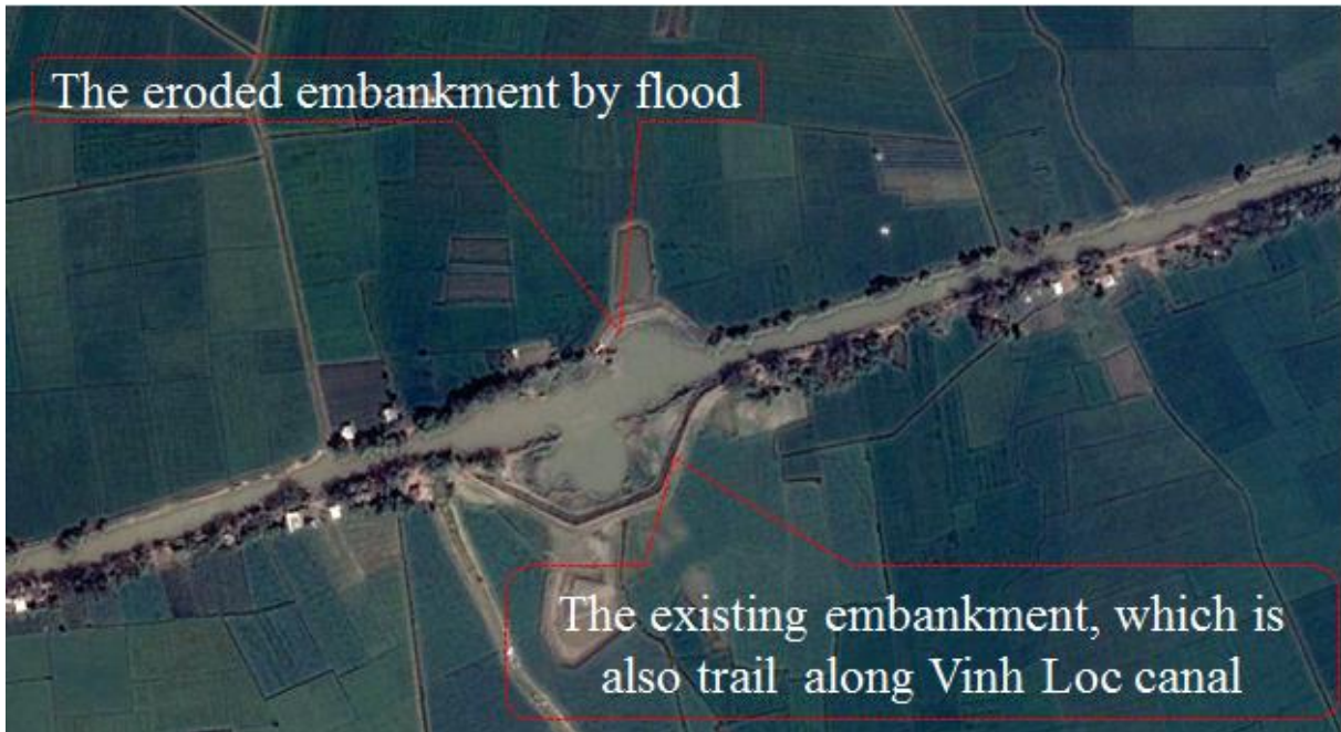
Figure 43: Erosion on Vinh Loc canal
