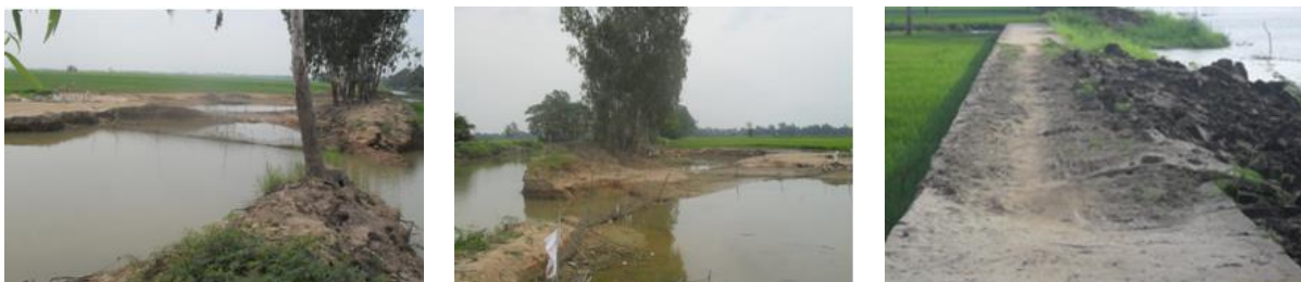
Figure 41: Erosion in the subproject area
