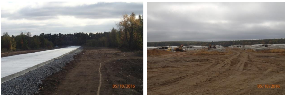
Figure 6.12 Concrete slab road deck after installation (left) and Brigade rearing sheds constructed from same pre-fabricated concrete slabs (right)
