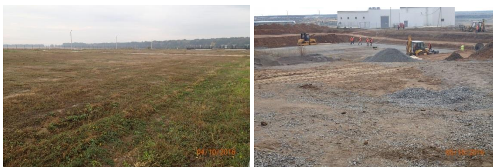
Figure 6.7 Baseline site conditions, Hatchery extension (left) and construction site WWTP extension (right)
