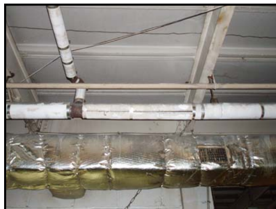
Photograph No. 12 – Piping with suspect asbestos containing material insulation.
