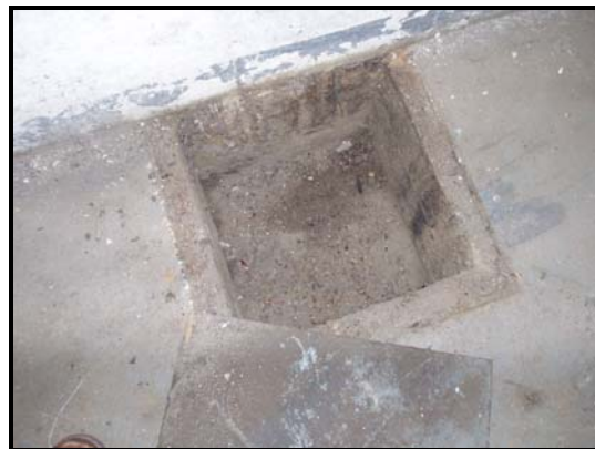
Photograph No. 6 – View of an interior floor drain with exposed soil bottom.
