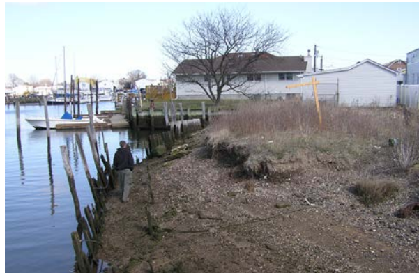
Shoreline erosion from increased severe storms is a threat to SGCN.
