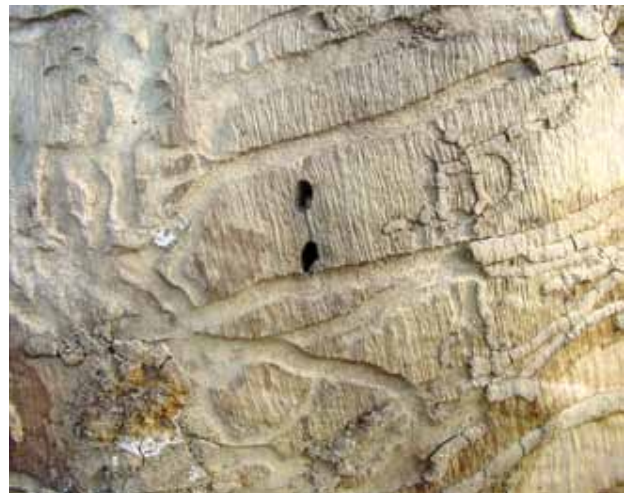
Figure 13. Close up of figure 12 showing holes tunneled into wood.
