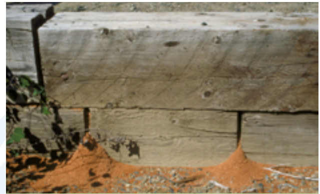
Carpenter ant damage (Edward H. Holsten, USDA Forest Service, Bugwood.org)
