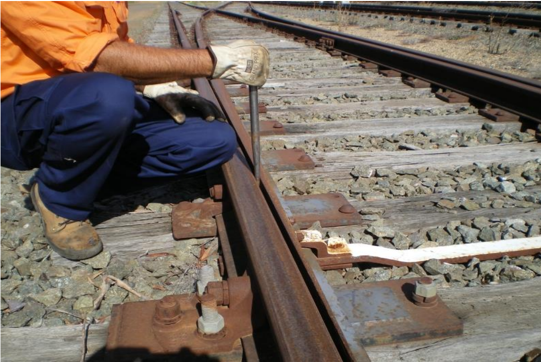
Photo 1 Checking Spring Lever Tension (manual operated points)
