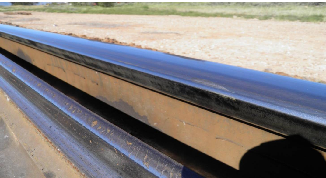
Photo 2 RCF Cracking on Head of Tangential Switch Blade
