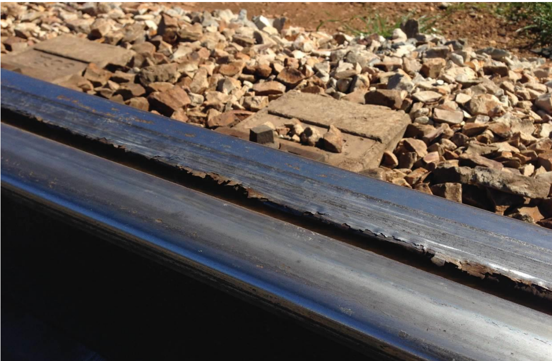
Photo 4 Damaged Stock Rail
