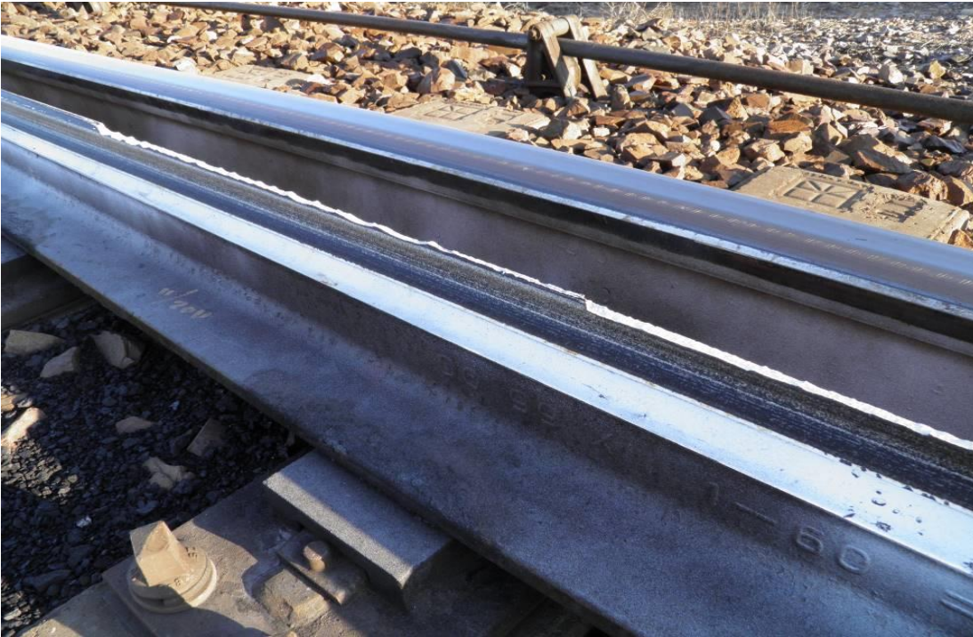
Photo 3 Switch Rail Head Damage Resulting from RCF Cracking
