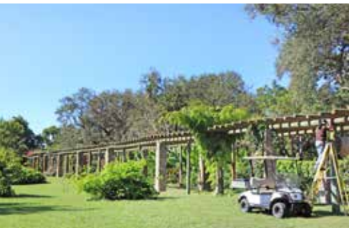
With the Pergola nearly complete as of this photo, vines were already twining their way to the top. Photo by Staff/FTBG
