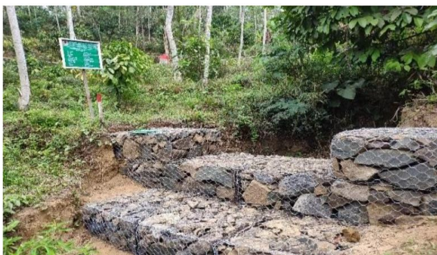
The installation of the retaining DAM is one of the RHL activities in a civil-technical way
