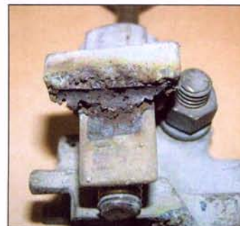
Figure 4: Buildup of contamination on clamping surface of hot tap in contact with copper conductor
