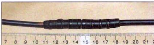
Figure 24: Macro image of compression splice on sample 4b. Note corrosion product on surface of conductor and splice
