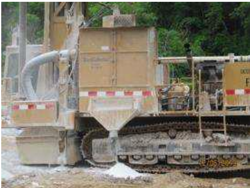
Figure 3.2 The dust collector on the drilling machine
