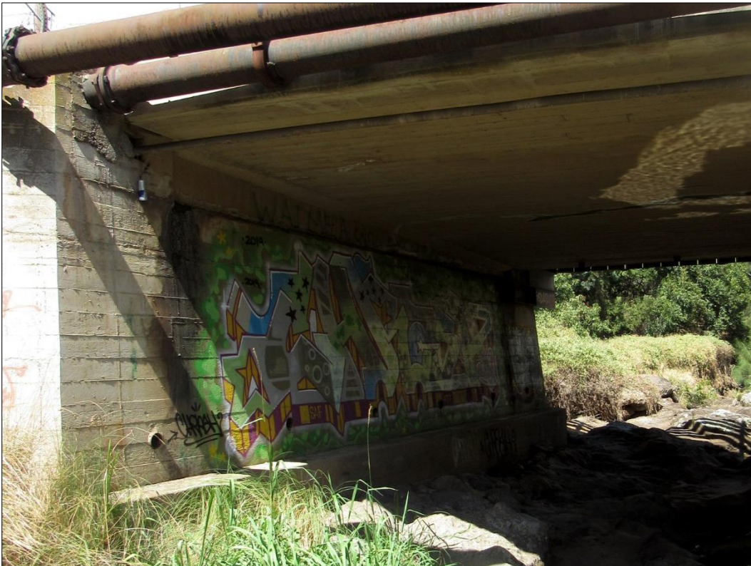
Figure 31. Site 29221 Waiaka Bridge detail of concrete abutment wall, view to the northwest.
