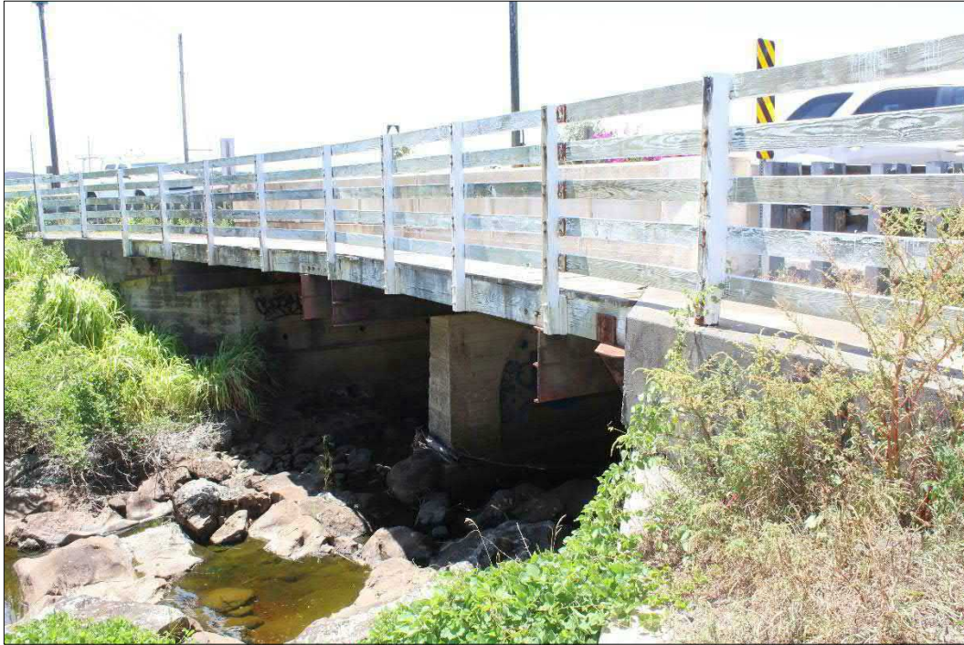
Figure 14. Waiaka Bridge with Keanu'imanō Stream below; traffic in background is traveling westbound; view towards southeast.
