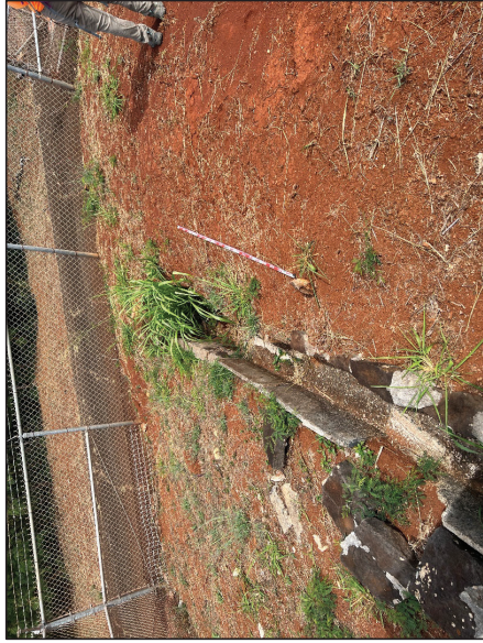
Figure 33. Photo I. Overview of the northern portion of the drainage culvert; note the mortared basalt sections of the culvert; view to north
