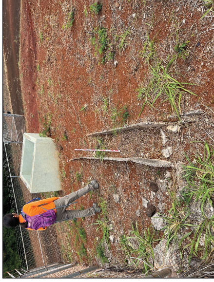
Figure 31. Photo G. Overview of the concrete drainage culvert and drain box; view to north
