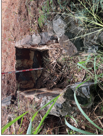
Figure 35. Photo K. Photograph showing the drainage culvert outside the project area; view to southeast
