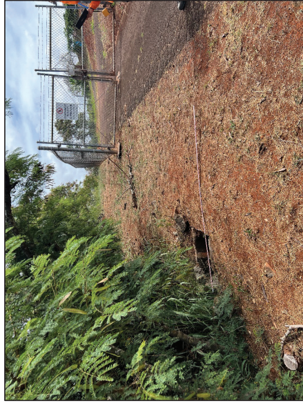
Figure 34. Photo J. Overview of the location of the drainage culvert outside the project area; view to northeast
