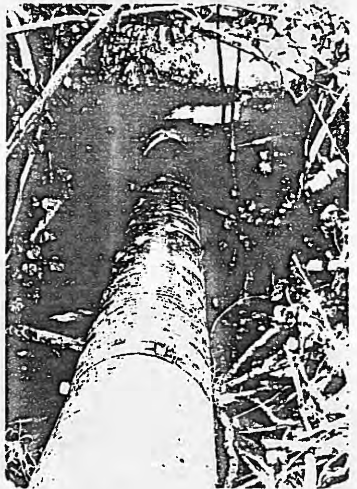
Short pipe section of Kuna Ditch.
