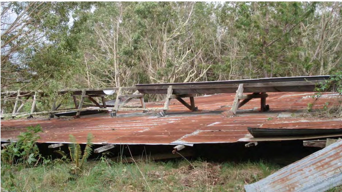
Figure 15. Gutters at the ends of the roofing material, view to the southeast.
