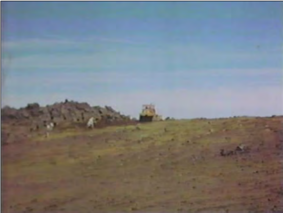
Screen capture from 1964 video showing the MSSS site being leveled by a bulldozer before construction.
