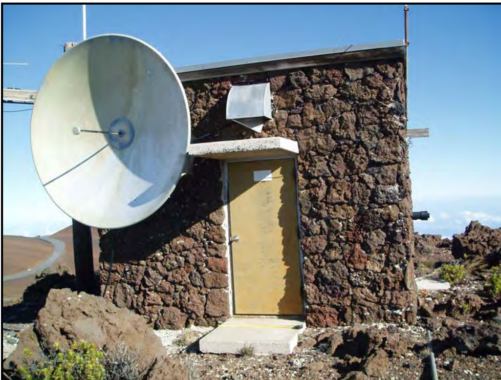
Photograph 12: General view to the north of Reber Circle of an older mid-1960s antenna building (see Figure 3 for location of this structure).
