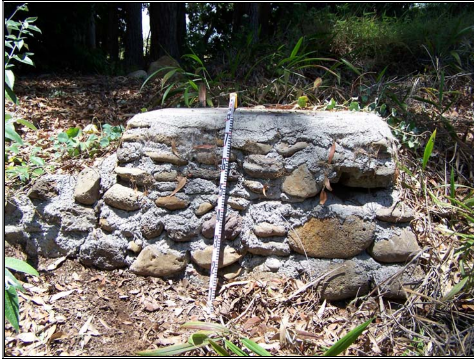
Figure 19. Modern pipeline support structure within the current project area, view to east
