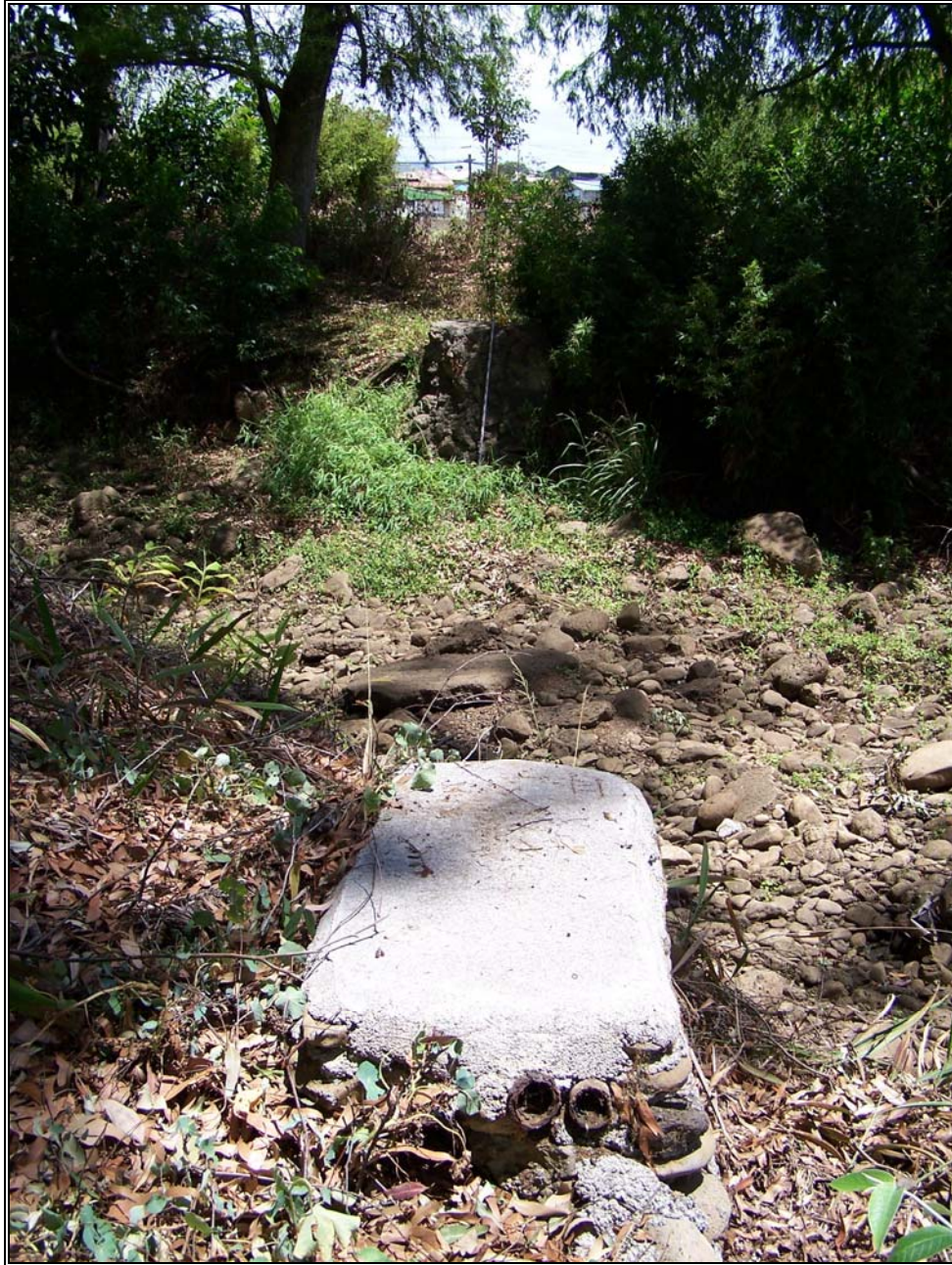
Figure 18. Two pipeline supports along Waikōloa Stream, view to south
