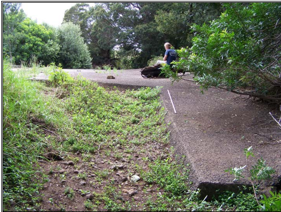
Figure 31. Eastern side of SIHP# -26873 showing concrete ramp and sediment-filled culvert opening, view to west
