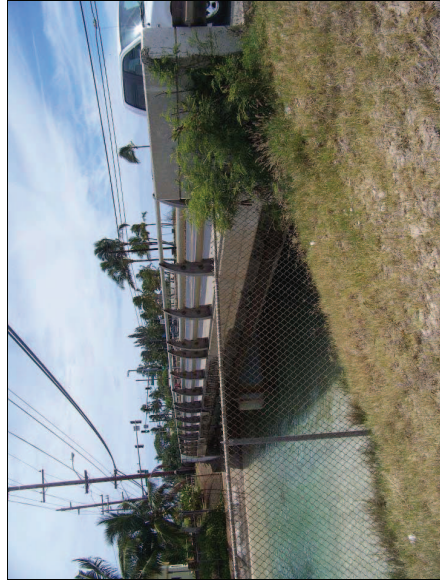
Figure 18. Photo of Maipalaoa Bridge and channelized drainage on the eastern side of the project area; view south
