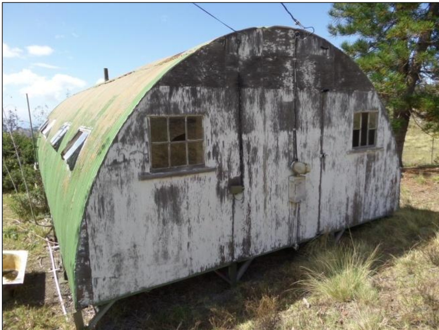
Figure 74. Southeast side of hut enclosed with wood framed wall and two windows, facing northwest.
