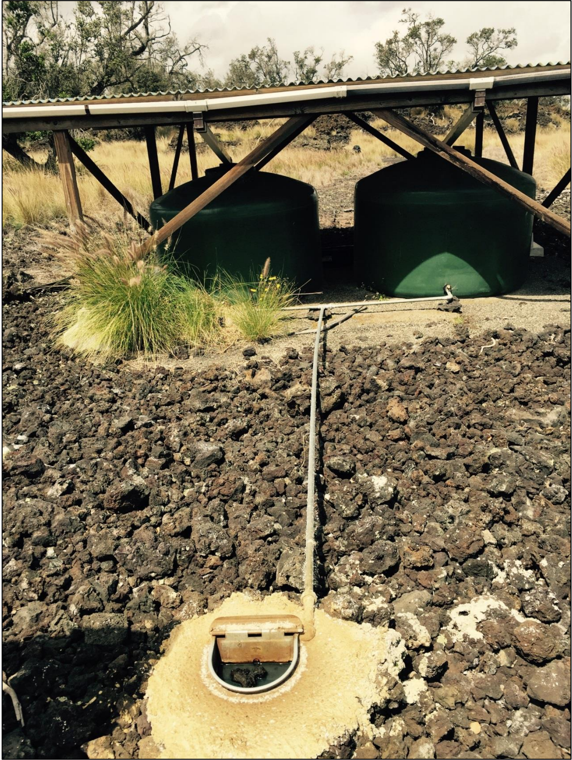
Figure 1.4 Game guzzler located in the PAHGMA. Float valve and trough in the foreground, connected to the catchment system pictured in the background.
