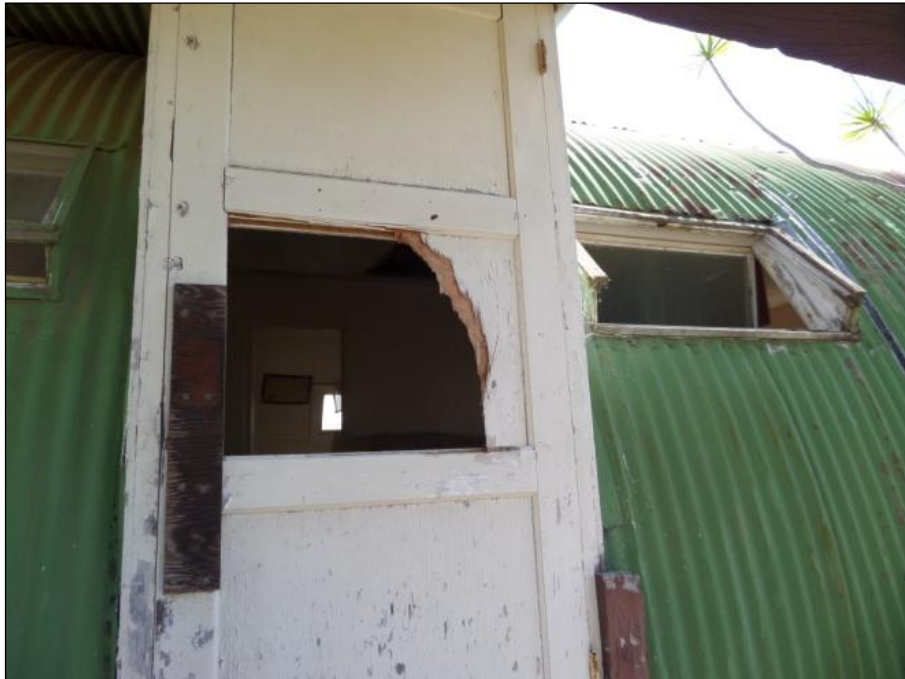
Figure 76. Broken door on northeast side of Quonset hut, facing southwest.
