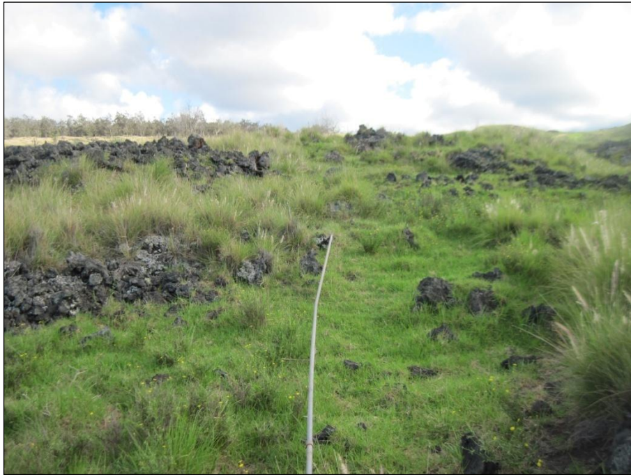
Figure 87. Galvanized water pipe running through Site 30307. View to south.
