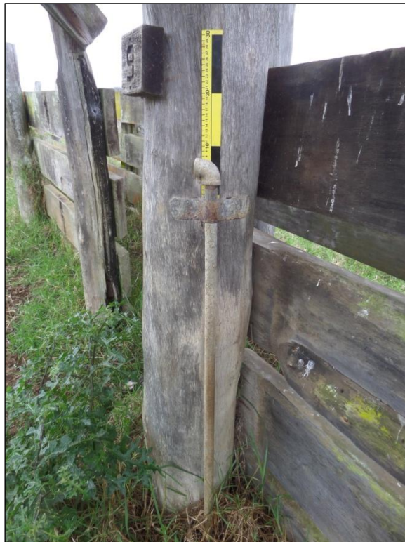
Figure 100. Close-up of engraved wooden marker and galvanized pipe waterline attached to support post of chute.
