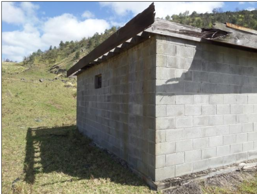
Figure 80. Northeast portion of quarry office with unpainted wall and wood joist ceiling.
