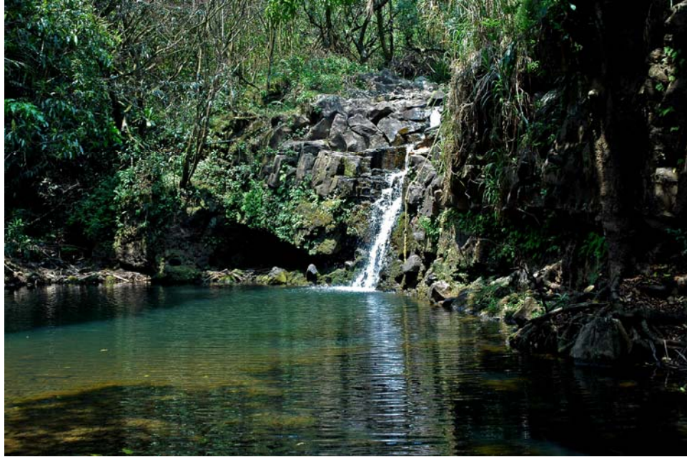
Large plunge pool below the three by-pass pipe diversion on Haiku diversion & ditch.
