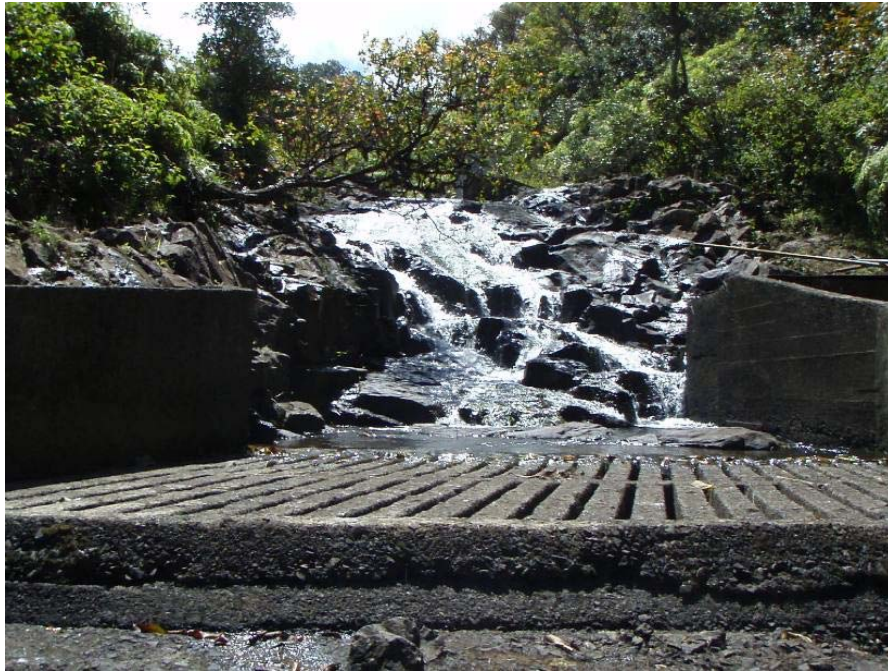
Looking upstream from below the first upper reach diversion on Honopou Stream. Image taken on 3/6/08.
