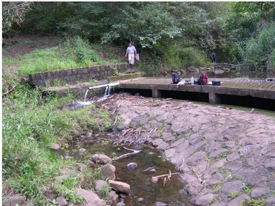
Water flows through three by-pass pipes across the Haiku diversion irrigation ditch. The pipes prevent the upstream movement of native amphidromous animals. An improved design eliminating the pipe overhang with water trickling down a continuous sloping hard surface might provide access upstream with no change in the amount of discharge.
