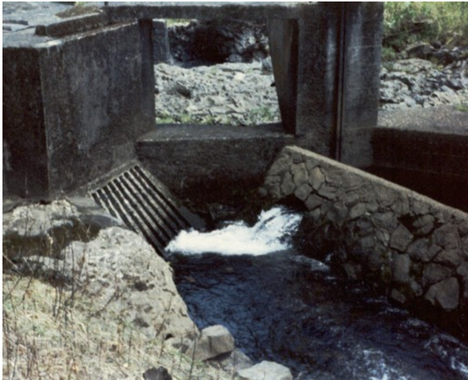
Figure 5-13. Diversion structure on the upper reach of Wailua Iki East Stream above Hāna Highway. (CWRM diversion photo 288.1).
