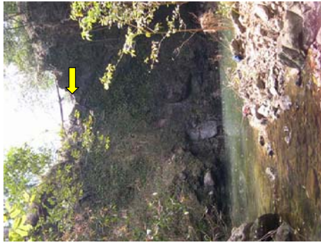
Upstream view of dry waterfall at site gh074r-030508. Note concrete diversion structure (yellow arrow) below fallen tree at the top of the cliff.
