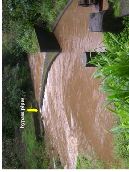
High flood waters over the irrigation ditch with the three bypass pipes. Note the lack of a simple passage way even at these high flows.
