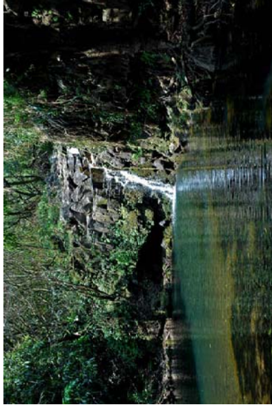
Large plunge pool below the three by-pass pipe diversion on Haiku diversion & ditch.
