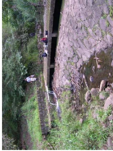
Water flows through three by-pass pipes across the Haiku diversion irrigation ditch. The pipes prevent the upstream movement of native amphidromous animals. An improved design eliminating the pipe overhang with water trickling down a continuous sloping hard surface might provide access upstream with no change in the amount of discharge.
