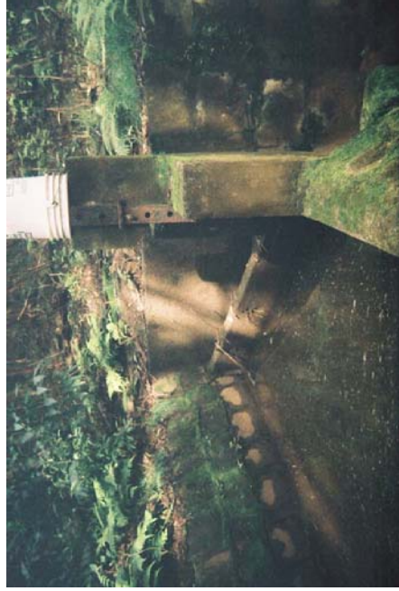
Better view of control gate.
