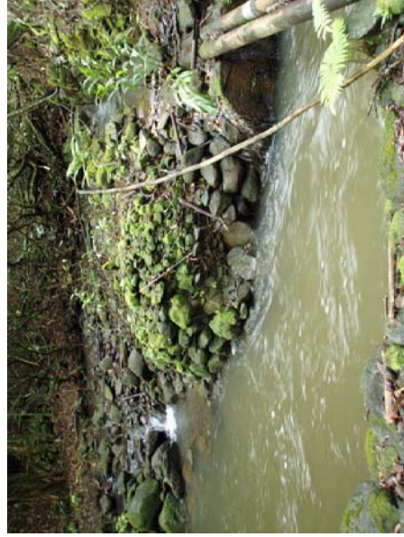
Note the two pipes on the right that pass over the ditch and transport water from stream. They are connected to one PVC pipe which empties back into the stream downstream.
