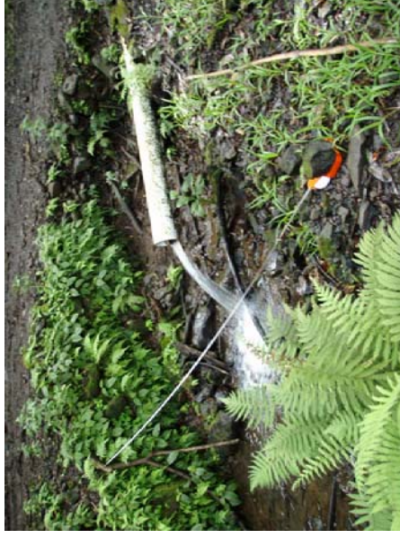
Pipe over Lowrie Irrigation ditch Hanehoi Stream (above Hana Highway and Ernie Schupp). Pipes make it difficult or impossible for upstream migration of native animals except at flood flows when the diversion is completely overtopped by the stream flow.
