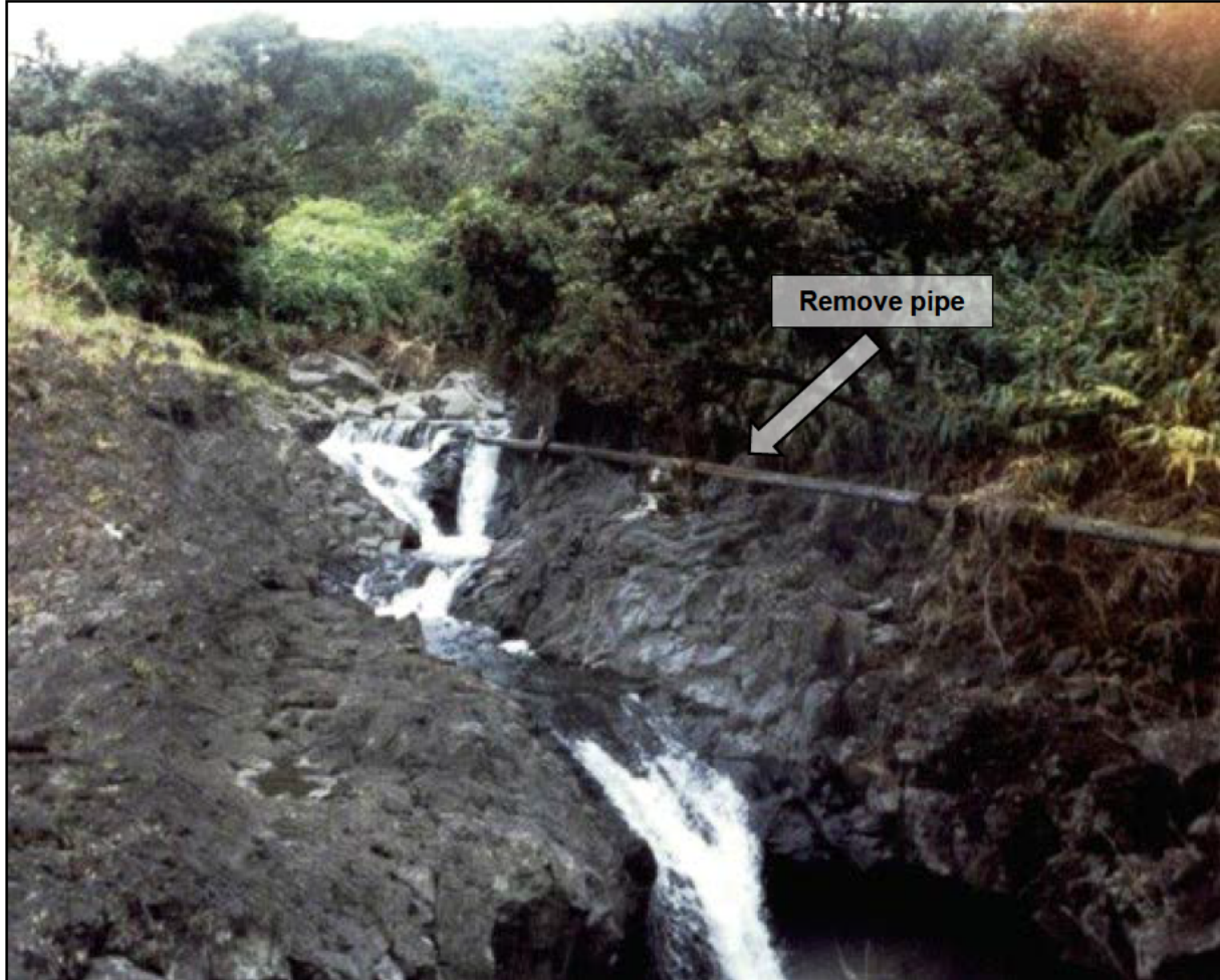
Photo 12. Pi'ina'au six-inch steel (and PVC) pipe at Ko'olau Ditch (K-31a) (1989).
