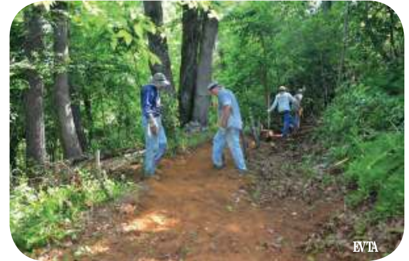
EVTA volunteers clearing a section of trail between Roaring Gap Road and Wells Knob Road.
