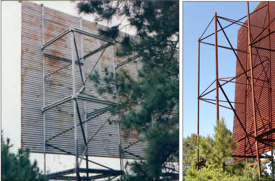
Figure 16: At Left, “Back of screen,” 1995 Photograph Submitted by Rick Hasley, Tower Drive-In Theatre, Rocky Mount, North Carolina. 65 At right, detail of Gaston Drive-In Theatre trellis.
