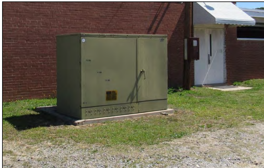
Photo 78: Electric Box, Southwest Oblique.
