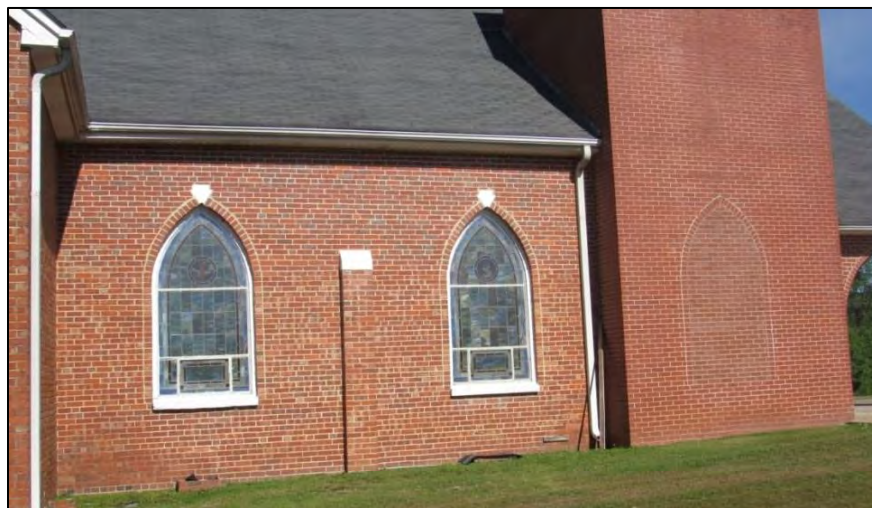
Photo 50: Windows on the Original Core (East Elevation) and the Filled-in Window on the Tower.
