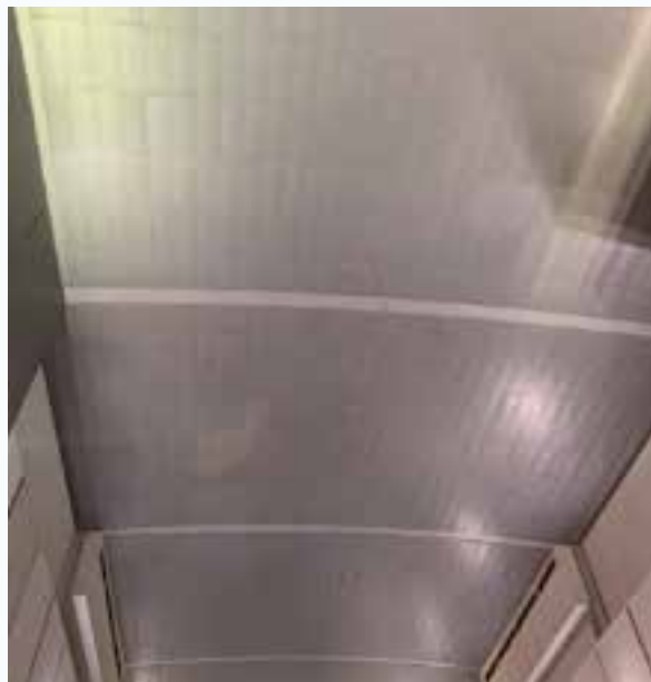
Figure 13 - Metallic perforated acoustic panels may become rust after some time (picture from Dubai's Airport), an issue that VMT technology can avoid, by ensuring the same look overtime.
