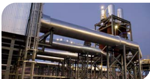
Wärtsilä has delivered a gas power plant to Nevada, USA.
