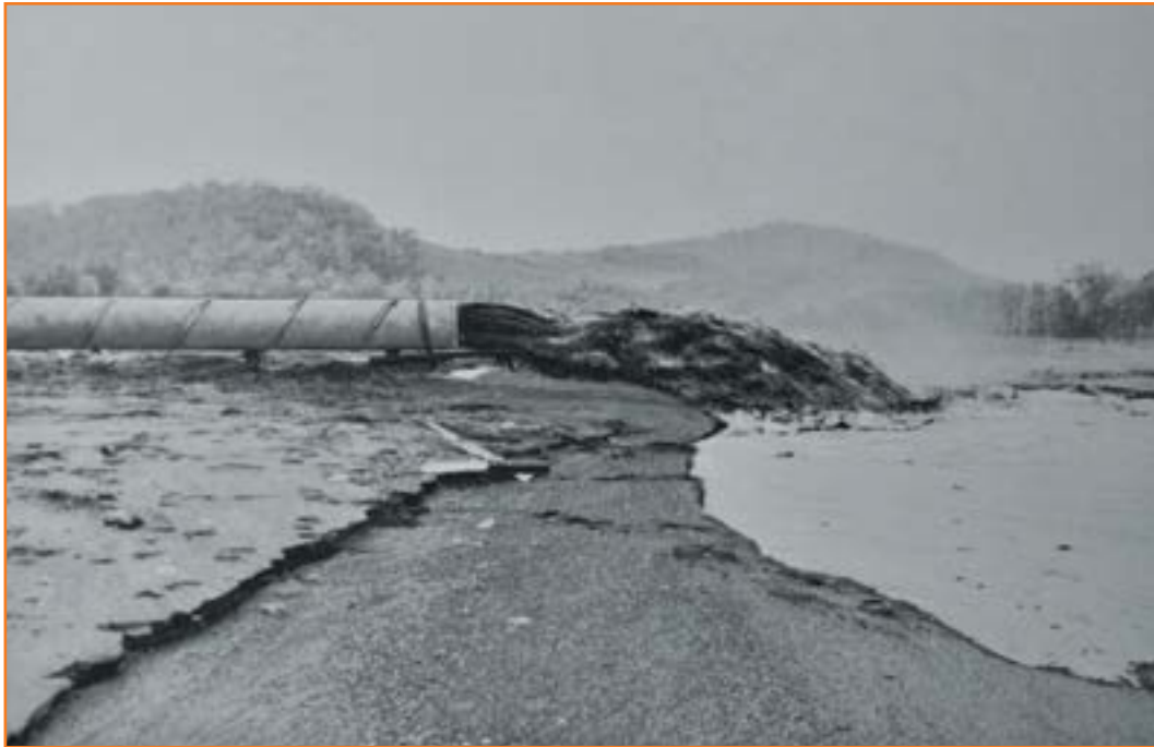
Figure 20.4 Schuylkill River desilting project discharging dredged materials into an impounding basin upstream at Stouds Ferry, Berks County. (From The Schuylkill River Desilting Project, Final Report of the Schuylkill River Project Engineers , 1 July 1951 17 )
