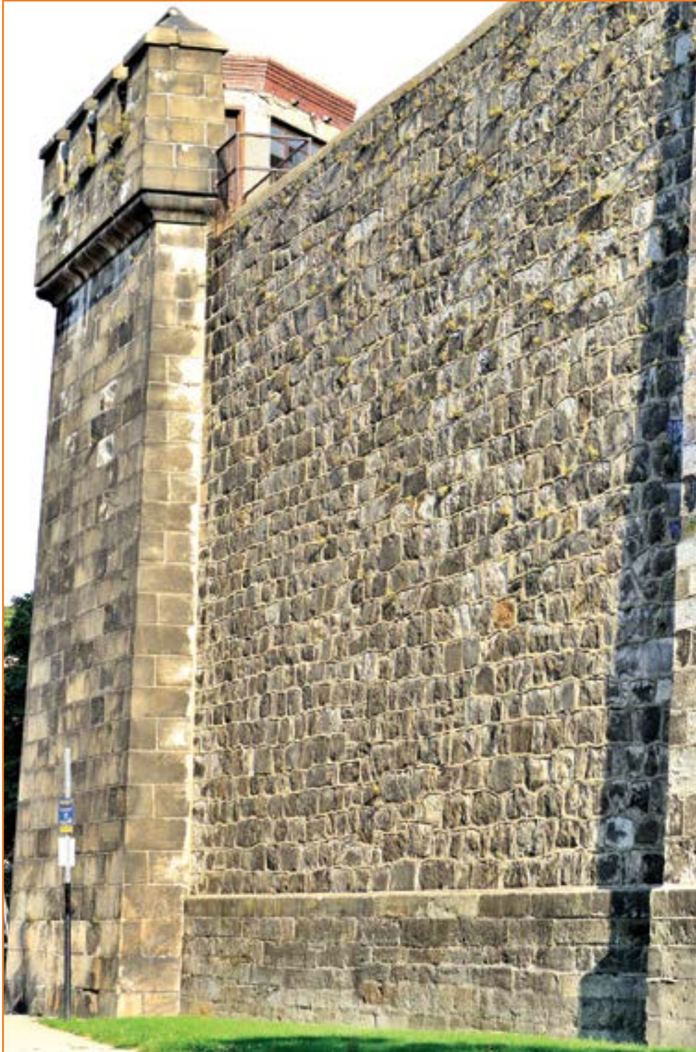
Figure 18.2 Eastern State Penitentiary, north wall, viewed looking east. At this distance, ferns growing in the wall are practically invisible.
