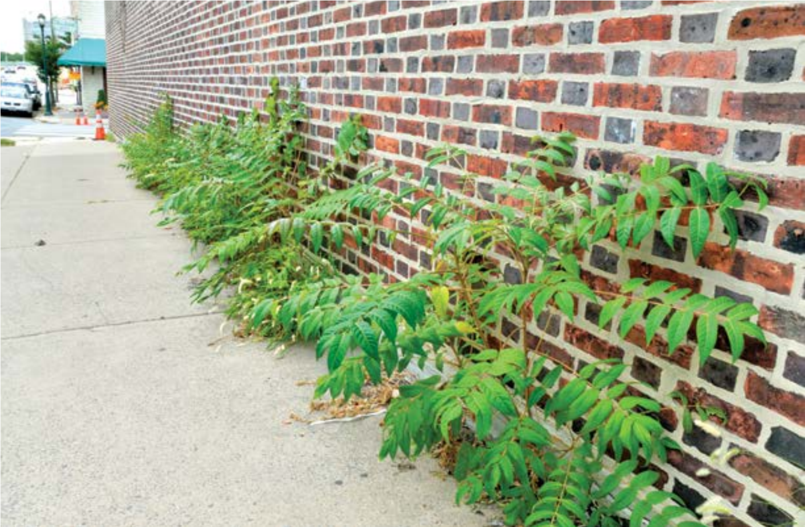
Figure 5.3 Colony of ailanthus saplings outside O'Connor Swimming Pool on Lombard Street. They are sprouting from roots tracking along the crack at the base of the wall.
