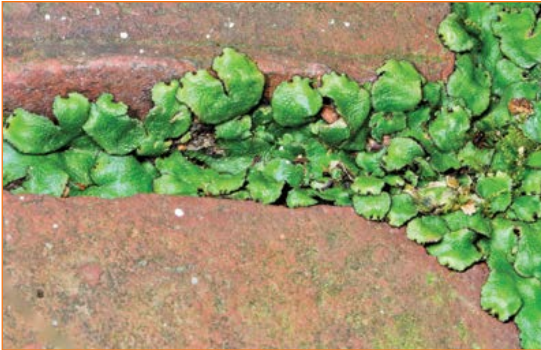
Figure 23.3 Reboulia hemaesphaerica between brick pavers.
