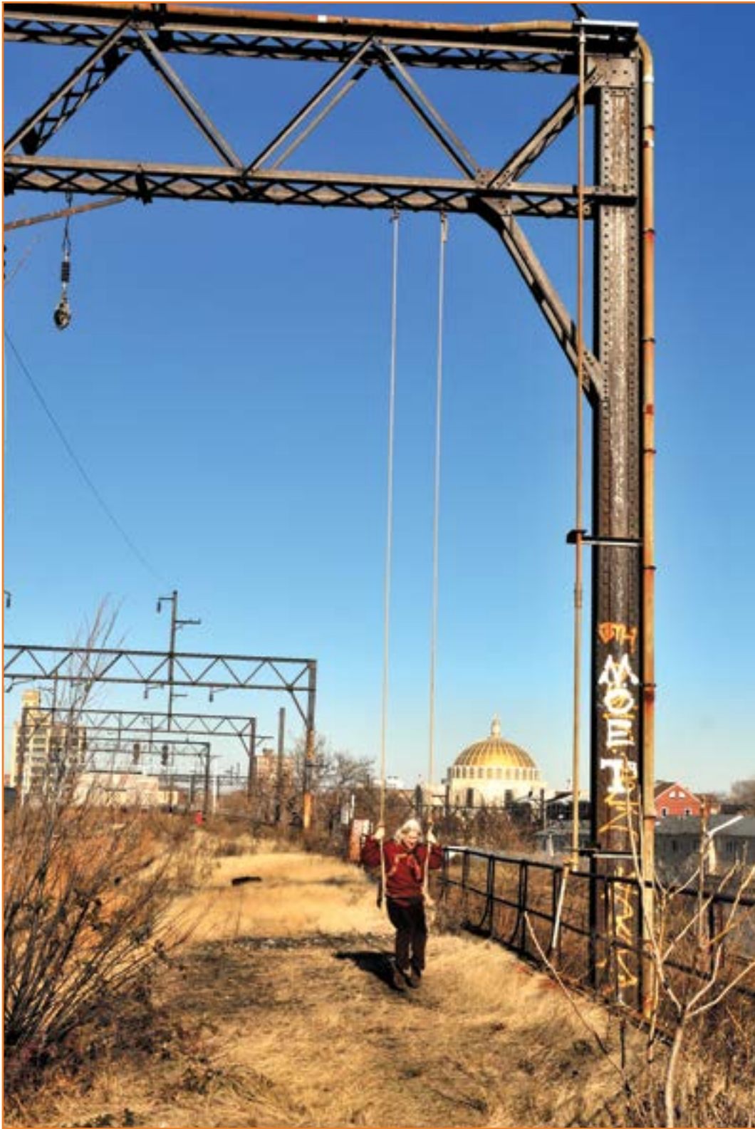
Figure 28.7 Reading Viaduct, December 11, 2011. Elevated above city streets, it carried trains into Reading Terminal Station from 1893 to 1984. In 1894, 290 trains on thirteen sets of tracks were scheduled to run daily from this station onto tracks such as those that once ran here. 34
