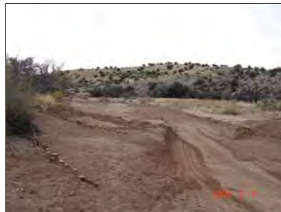
Fig. 4. Compound post vanes (set of three) slow water and force it to meander rightward and reconnect with the historic waterway.
