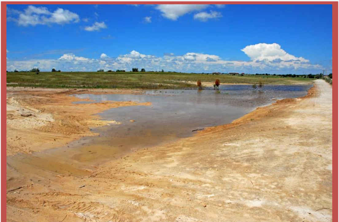
Ciénega cut and fill to redirect the Bass Lake Spring run along River Road. Bare soil and new microrelief may be suitable habitat for Pecos sunflower, but will also encourage exotic tree infestation.
