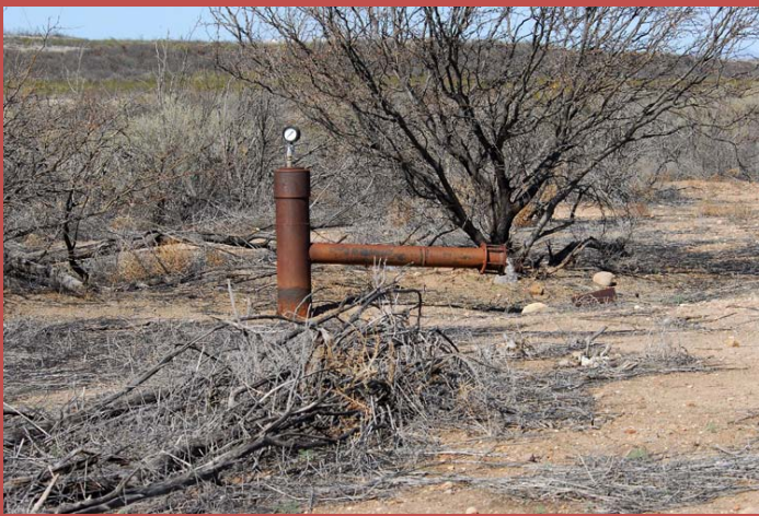
Abandoned irrigation well head at San Bernardino Ciénega.
