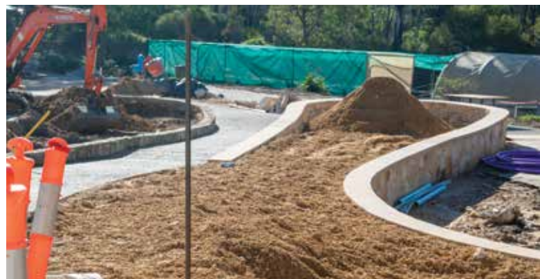
Soil replaced in new garden and in the distance excavating existing heavy soil from old garden beds
