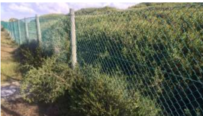
Figure 54. Vegetation growing through fence.
