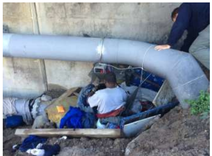
Figure 40. Illegal occupations under the Blaauwberg Road bridge.
