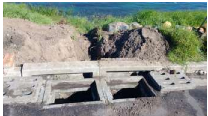
Figure 55. Internal stormwater drain that collapsed.
