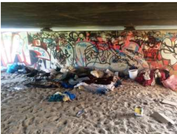
Figure 39. Illegal occupations under Otto du Plessis Drive bridge near Paddocks complex.
