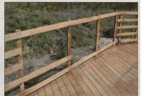
Panel have been broken off the bridge.
