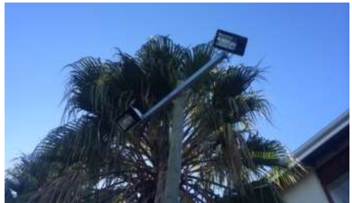
Figure 51. Security floodlight at entrance gate.
