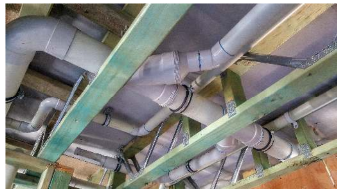
Figure 5: Trusses designed with allowances for services Courtesy of Independent Timber Supplies & Homebuys
