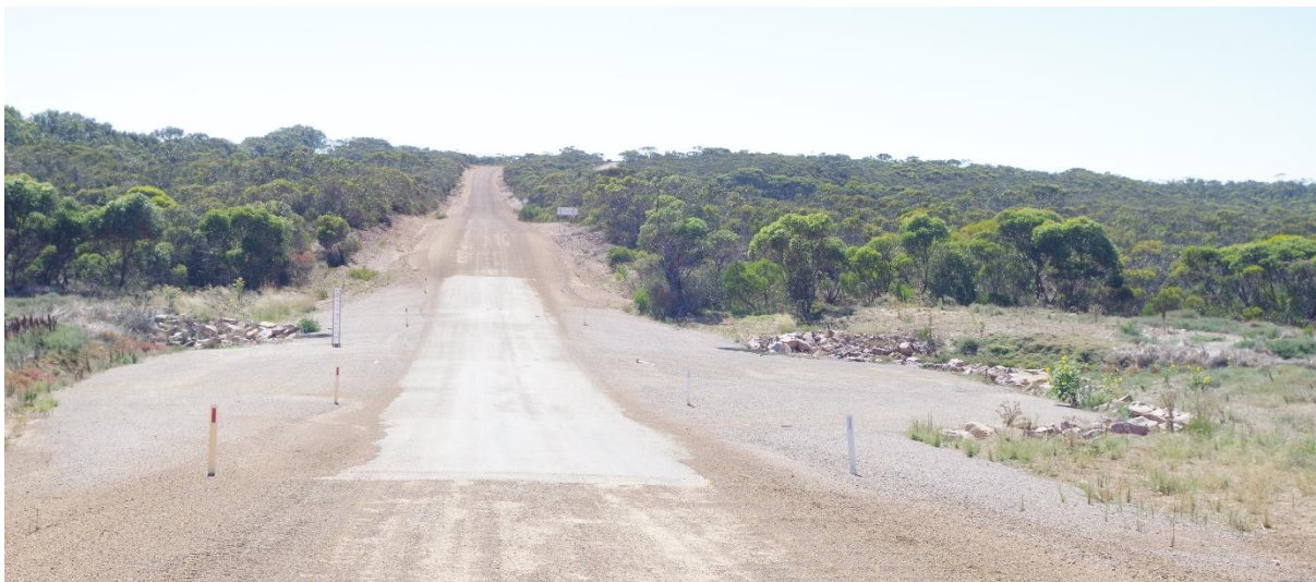
Figure 3. Road design along Neds Corner Rd at minor creek-line crossing been particularly shaped to allow free water flow and not interrupt hydrological water flows. Photo taken facing in a northerly direction.
