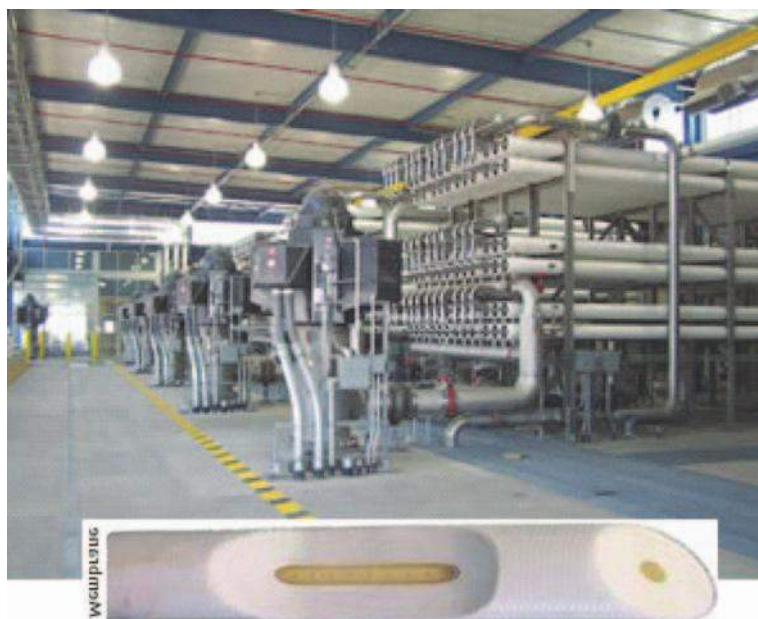
Figure 4 Membrane desalination plant. RO membrane units from El Paso Desalination Plant, Texas: the site of the world's largest inland desalination plant ( 104\,000\text{ m}^3\text{ d}^{-1} ). Production costs for water are less than less than 0.36\text{ \$ m}^{-3} . From http://www.epwu.org/167080115 .
