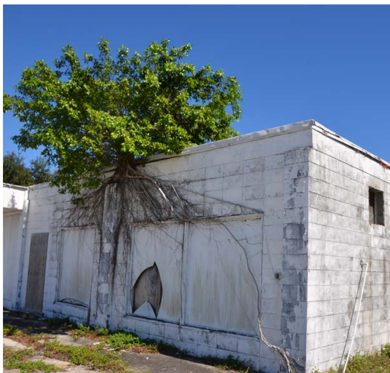
A F. microcarpa epiphyte on the roof and wall of an abandon building.
