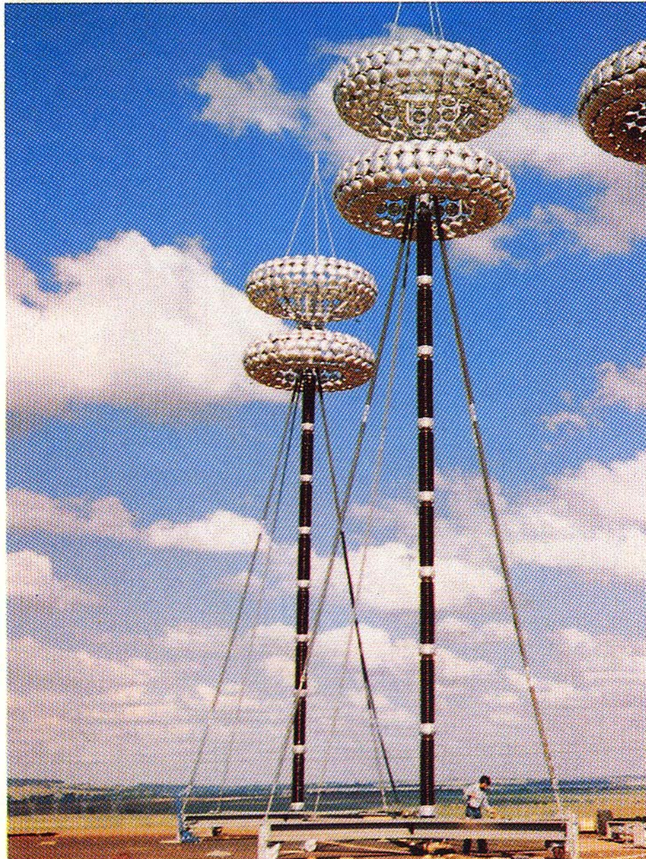
Large outdoor impulse voltage dividers, damped capacitive type with large top electrode for ultra-high switching impulse voltages
