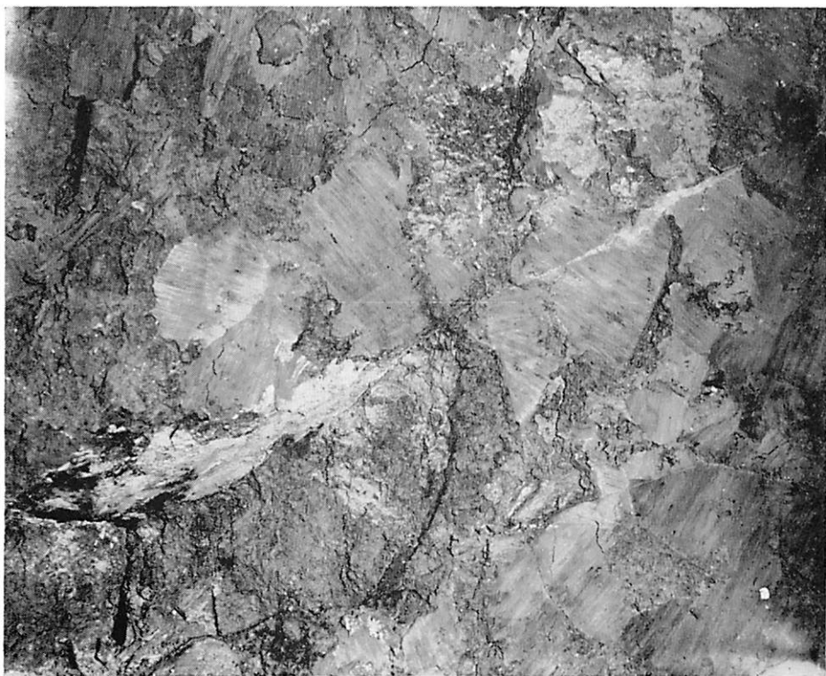
Figure 4.—Diagonally-filled crack in the wall of the pit at Eliza Clark School.
