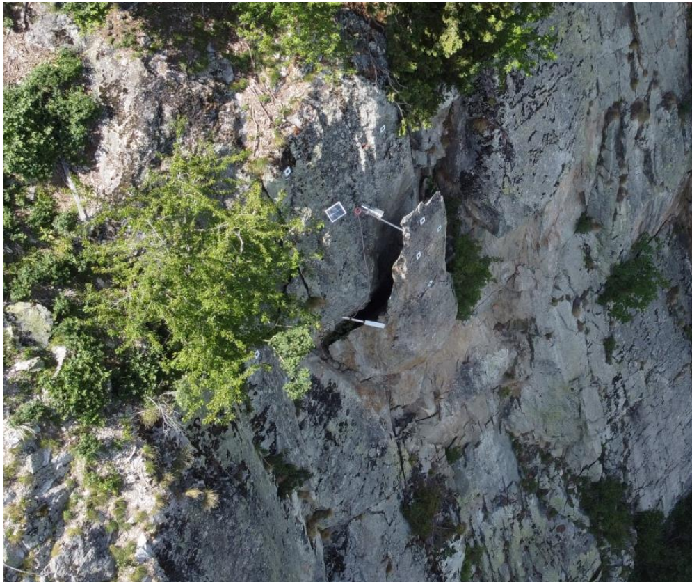
Figure 2. Overview of the monitored rock sheet (drone image). 9 targets (white squares) were installed on the moving (5) and stable (4) parts. The solar panel is used to power both extensometers (metal bars) visible along the back crack.
