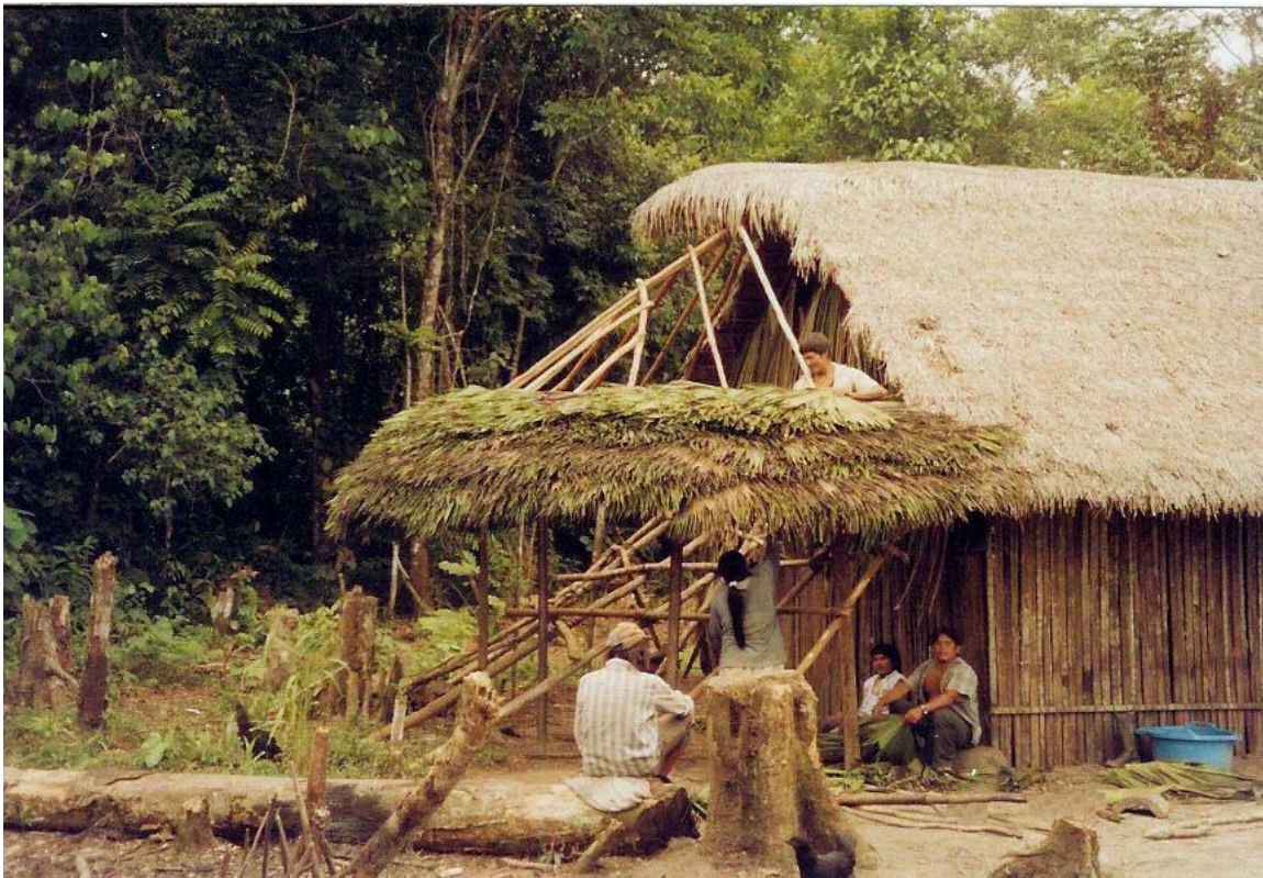
Figure 6.2 – An Aguaruna man and his family and friends are adding palm leaves to the roof of his house, Bajo Cachiaco.
