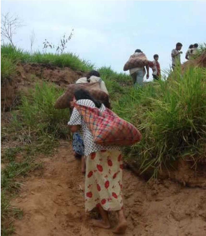
Figure 4.9 Tsimane' parents helping carry cement from the local "port" to the school construction site in Ivasichi. This voluntary work was done with the aim of having the school repaired before the rainy season.
